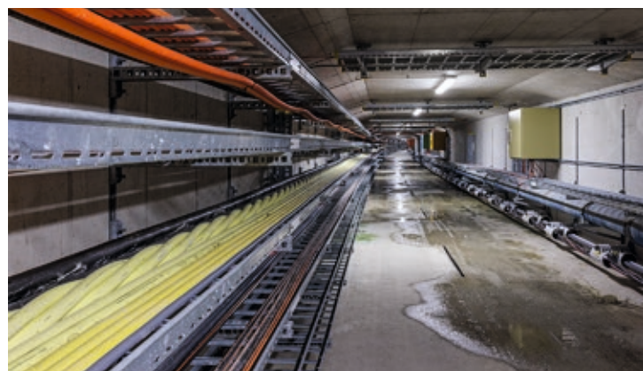
The service duct for the third Gubrist tunnel tube: disruptions in supply chains for special materials may affect the installation and progress of the work.
