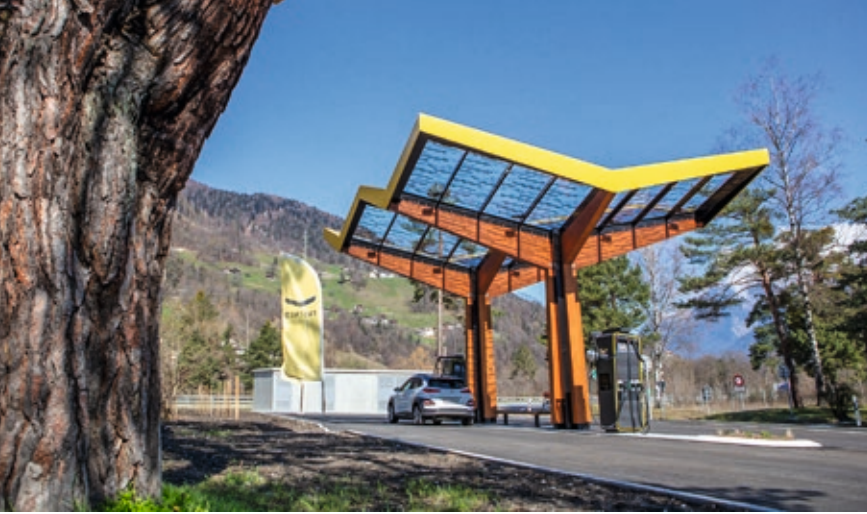
The fast charging station at the Apfelwuhr-Nord motorway rest area near Landquart (canton of Graubünden).
