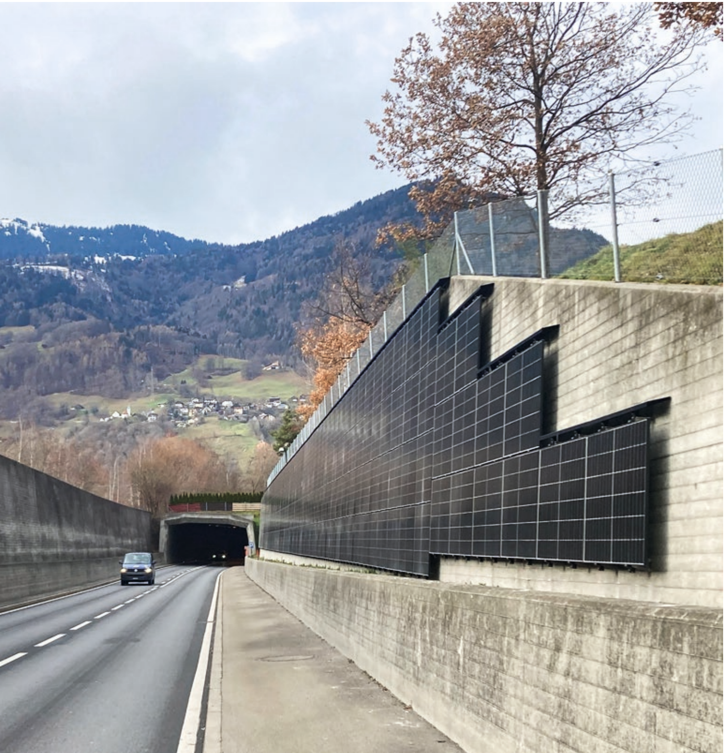
The solar panel installation at the eastern portal of the Karlihof tunnel on the N28 near Landquart (canton of Graubünden).
